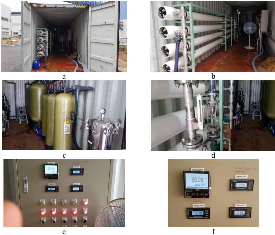
Figure 8. Example of a modular desalination system
