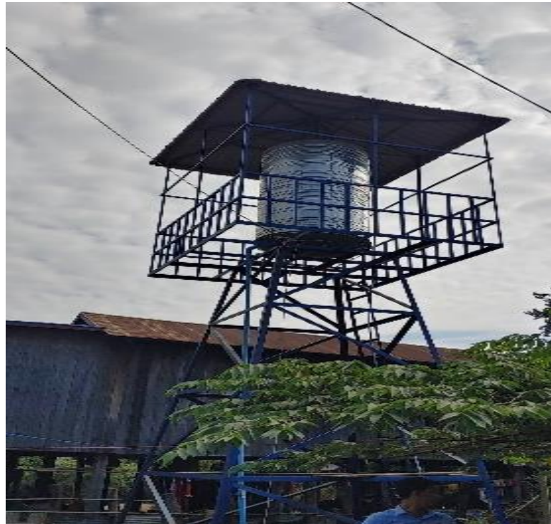
Photo 1: Installed water tank facility in the community
