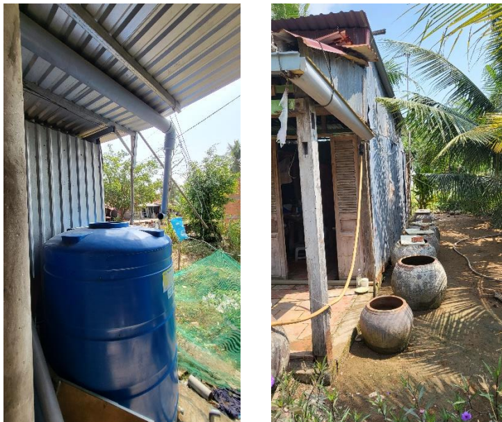
Figure 11. Water tank for collection of rainwater from rooftop.
